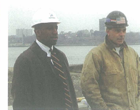
Robert Balachandran, left, surveys Pier 46 construction with Jim McLaughlin of Weeks Marine.
