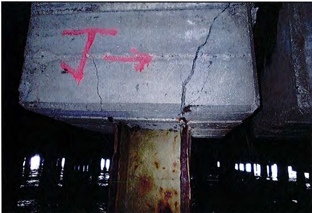
Photo B-14: Typical rust staining and delamination of epoxy coating at Bent Q.25, Pile Row 16S. Note, corrosion of the H-pile flange has caused a large crack in the concrete pile cap.
