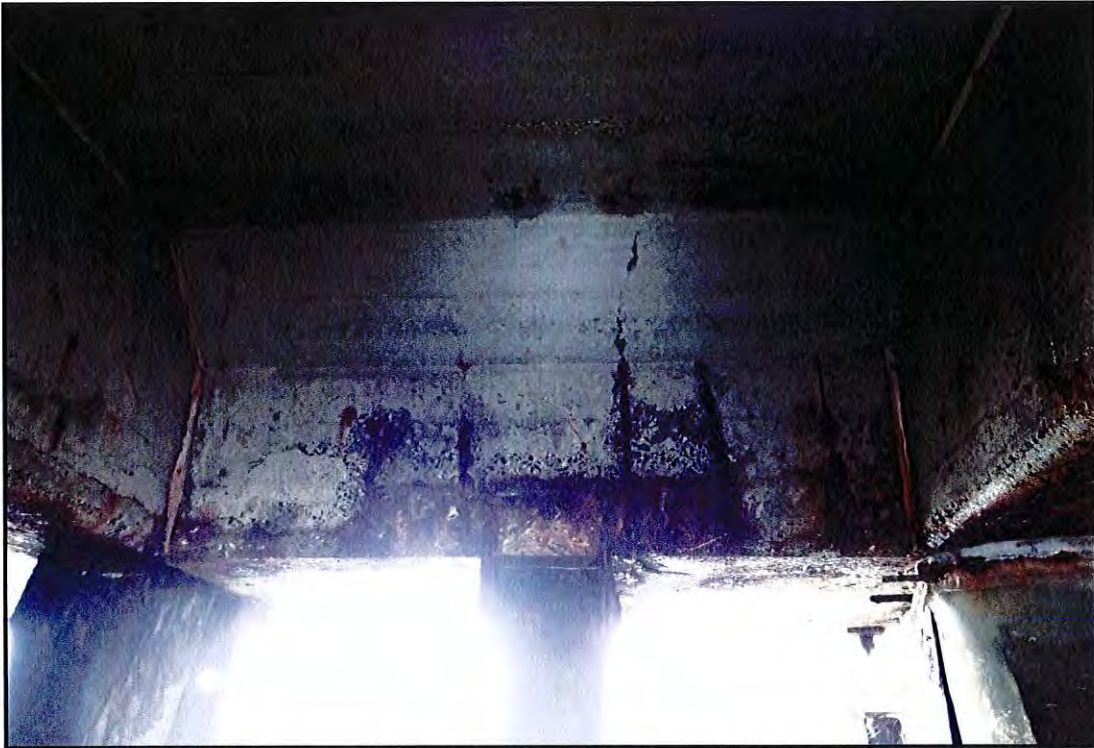
Photo B-37: Spall along the north cap of the Finger Pier Extension between Bent Z and Bent Z.2. View looking north.
