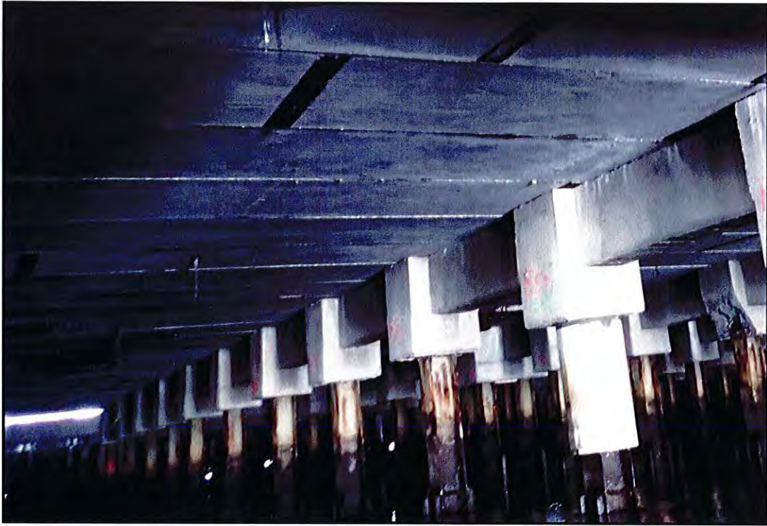
Photo B-3: View of typical Pier Shed substructure, looking north at Bent F-bar.
