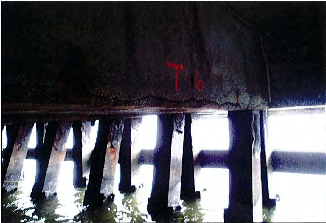
Photo B-5: View of typical Finger Pier Extension substructure, looking south at the southern edge beam of the pier.
