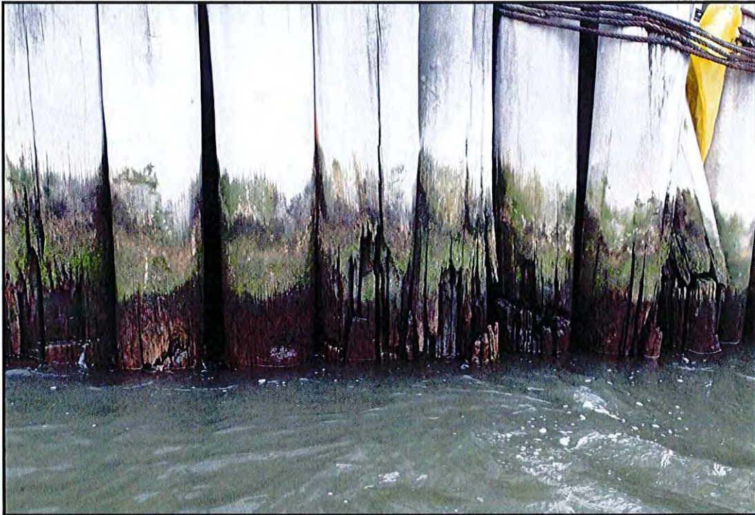
Photo B-41: Close-up of broken piles in the fender pile cluster at the north corner of the Finger Pier Extension.
