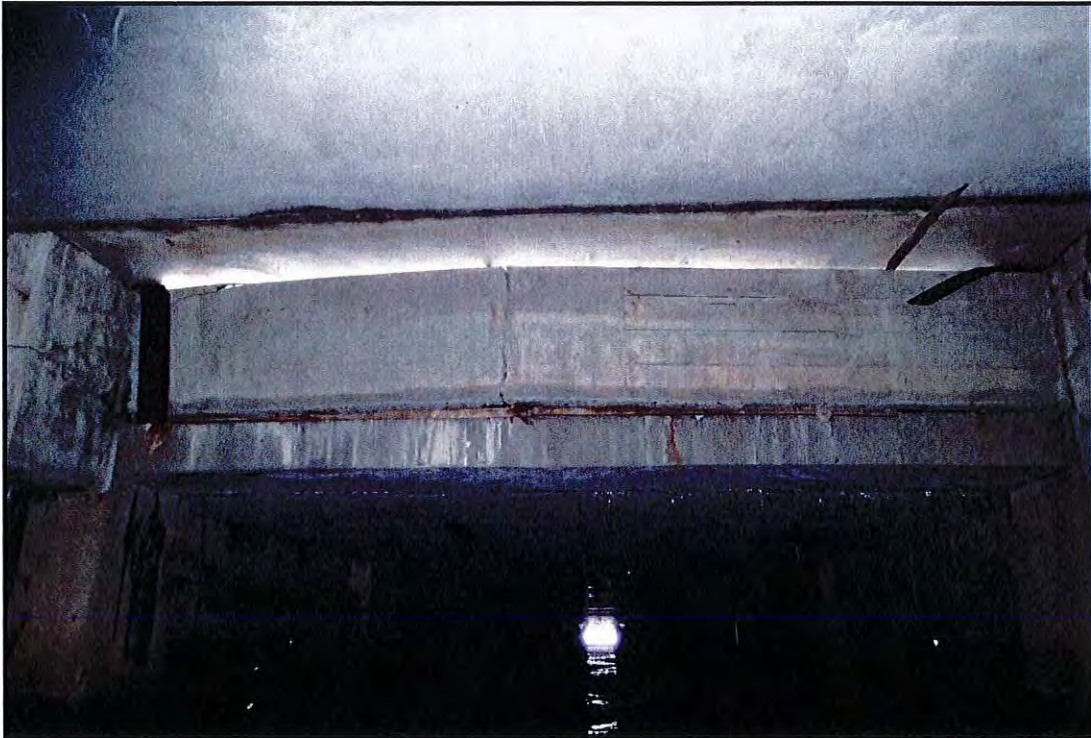
Photo B-29: Concrete closure wall with large vertical crack and deflection View looking north at Pile Row 7-bar between Bent I and I-bar.
