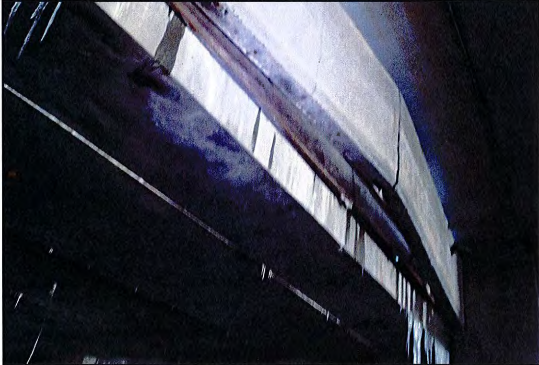
Photo B-30: Concrete closure wall with large vertical crack and deflection View looking east at Pile Row 7-bar between Bent I and I-bar.
