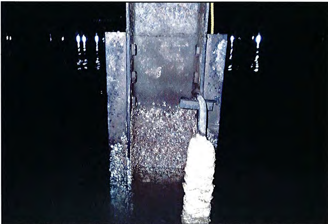
Photo B-12: Typical C-channel pile repair bolted to the flanges of H-pile I-bar 9-bar, view looking south.
