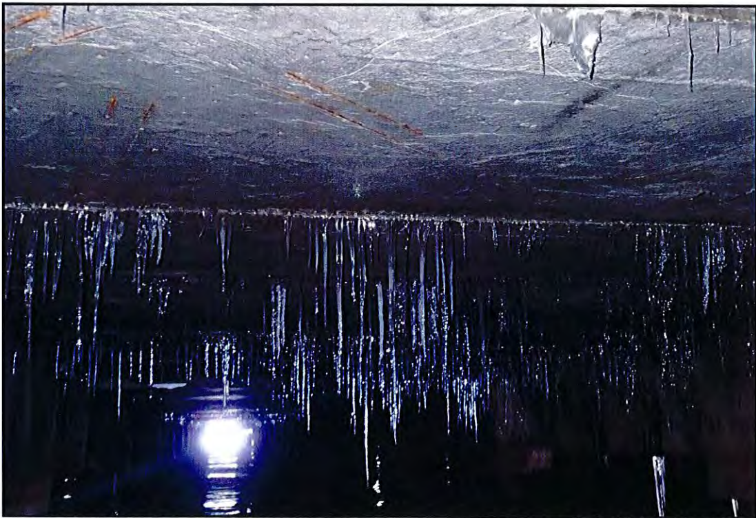
Photo B-4: Typical Court Yard substructure. Note water seeping through deck planks at icicle location.
