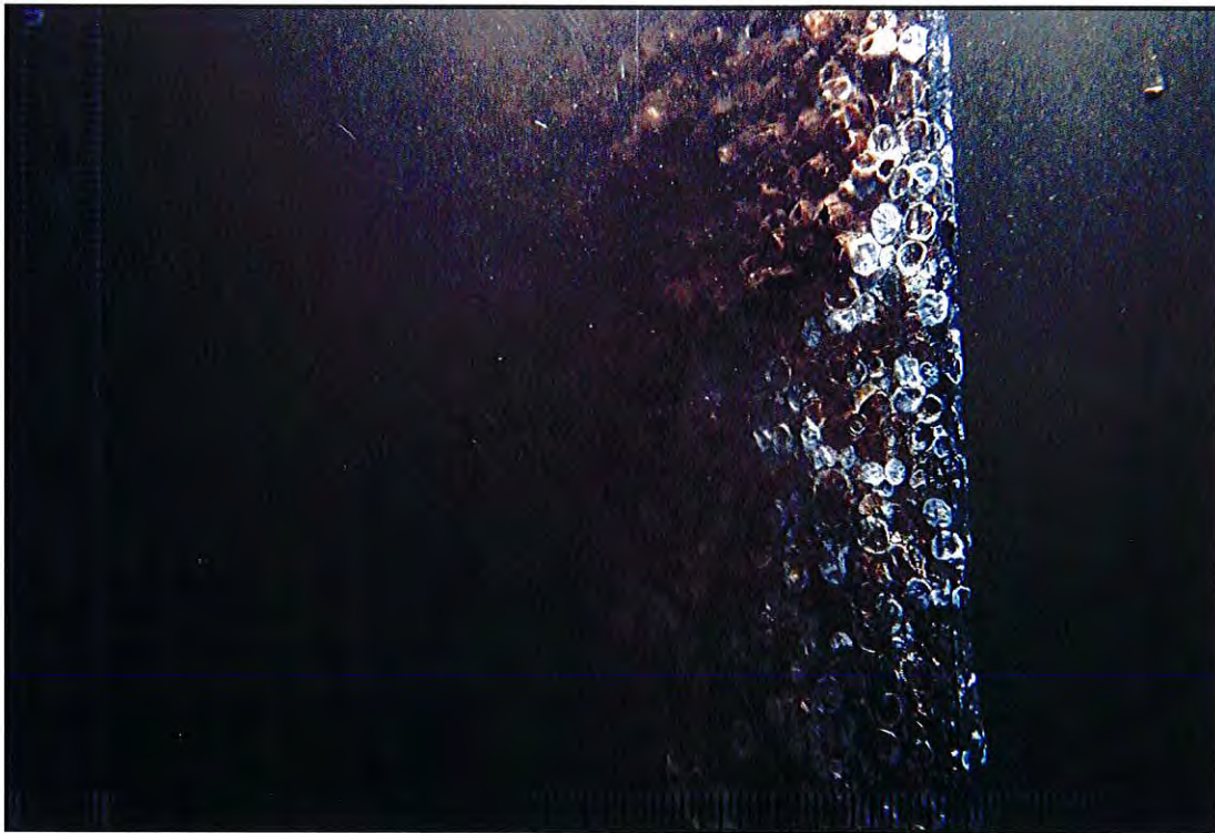
Photo B-19: Typical condition of the flange edge and flange face of a H-pile graded Major. H-pile location is the center-west H-pile of the pile cluster at Bent L and Pile Row 19.
