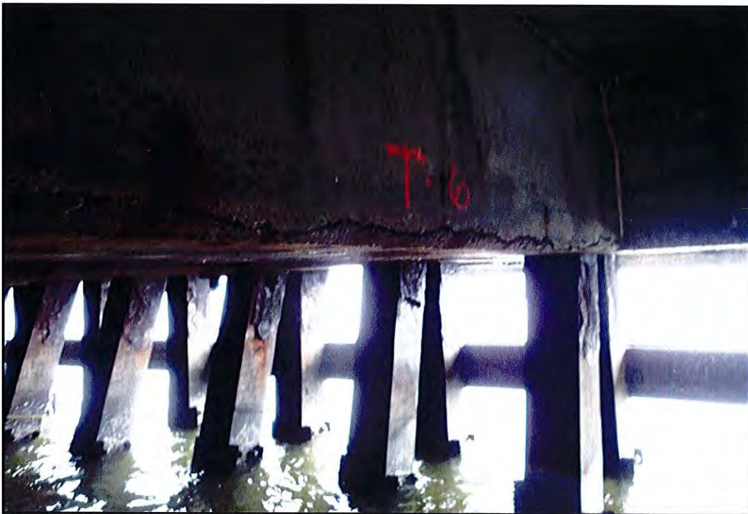
Photo B-32: Rust staining and delamination of the soffit of the first transverse beam north of Bent W at the Finger Pier Extension.
