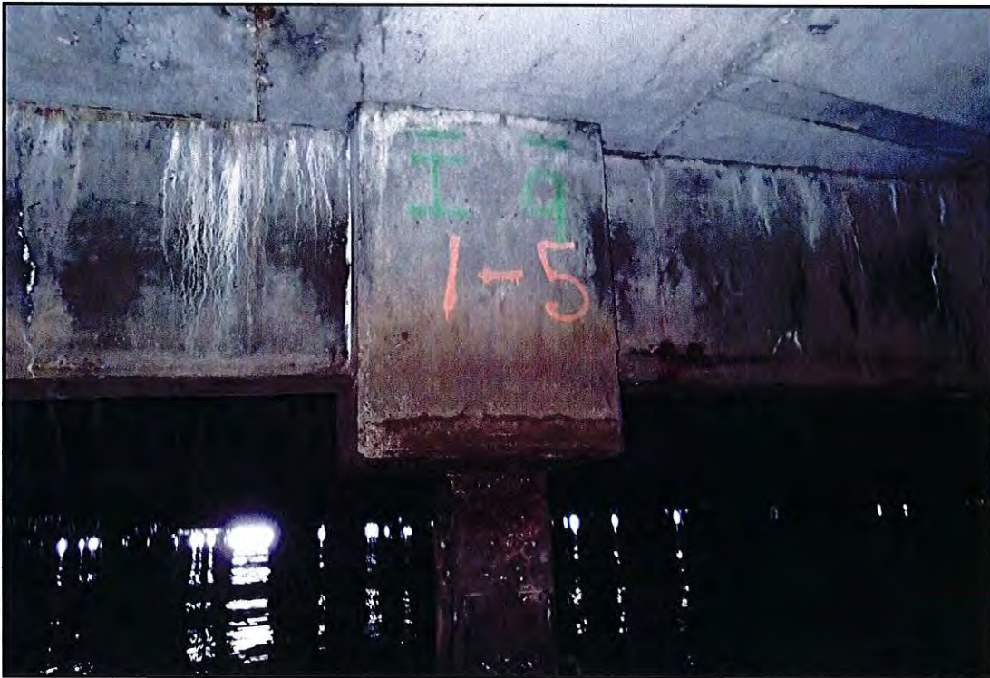
Photo B-24: Typical condition of concrete pile cap in the Court Yard. View looking west at Bent 1-bar, Pile Row 9-bar.
