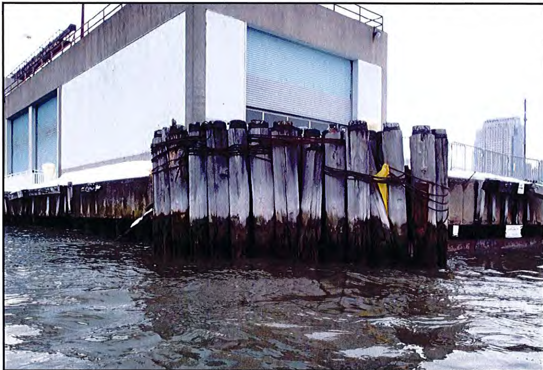
Photo B-40: Pile cluster at the north corner of the Finger Pier Extension. Note the severe damage at the MLW elevation and the loose wire rope wraps at the top of the cluster.
