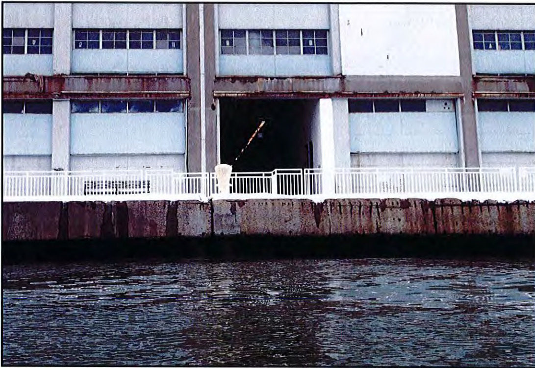
Photo B-31: Erosion up to 1 in. deep and exposed reinforcing along the full height of the western edge beam between Pile Rows 7 and 8-bar.
