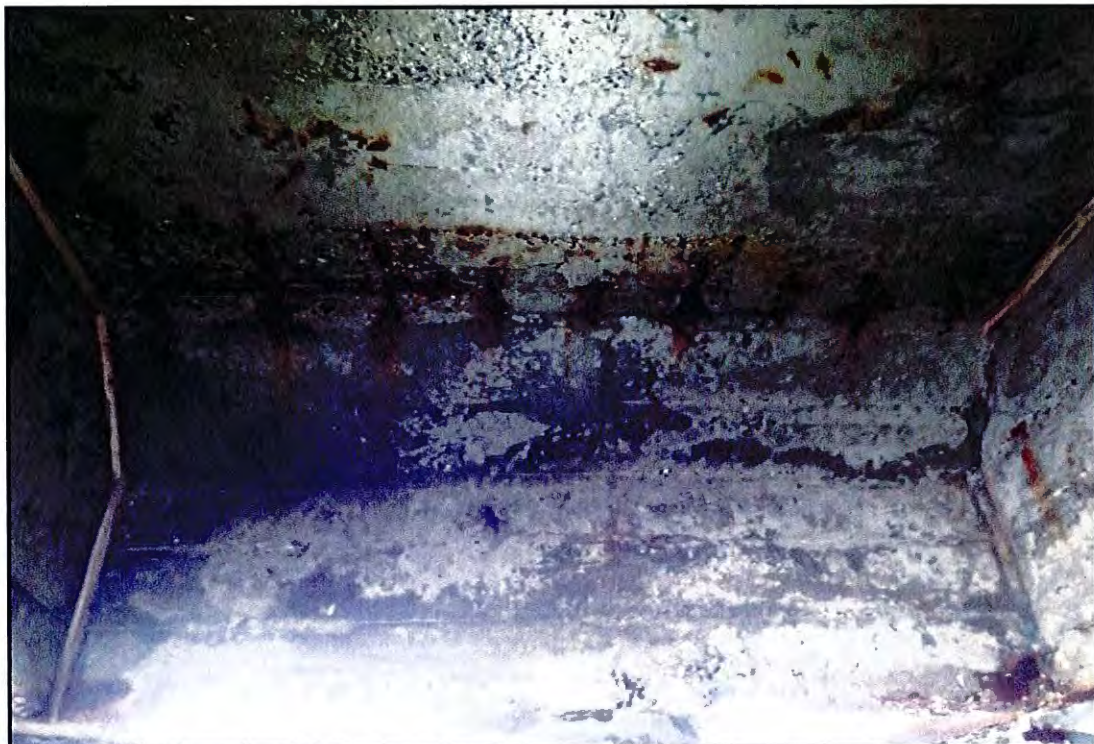
Photo B-38: Spall along the deck soffit of the Finger Pier Extension between Bent X.7 and Bent Y adjacent to the north cap. View looking north.
