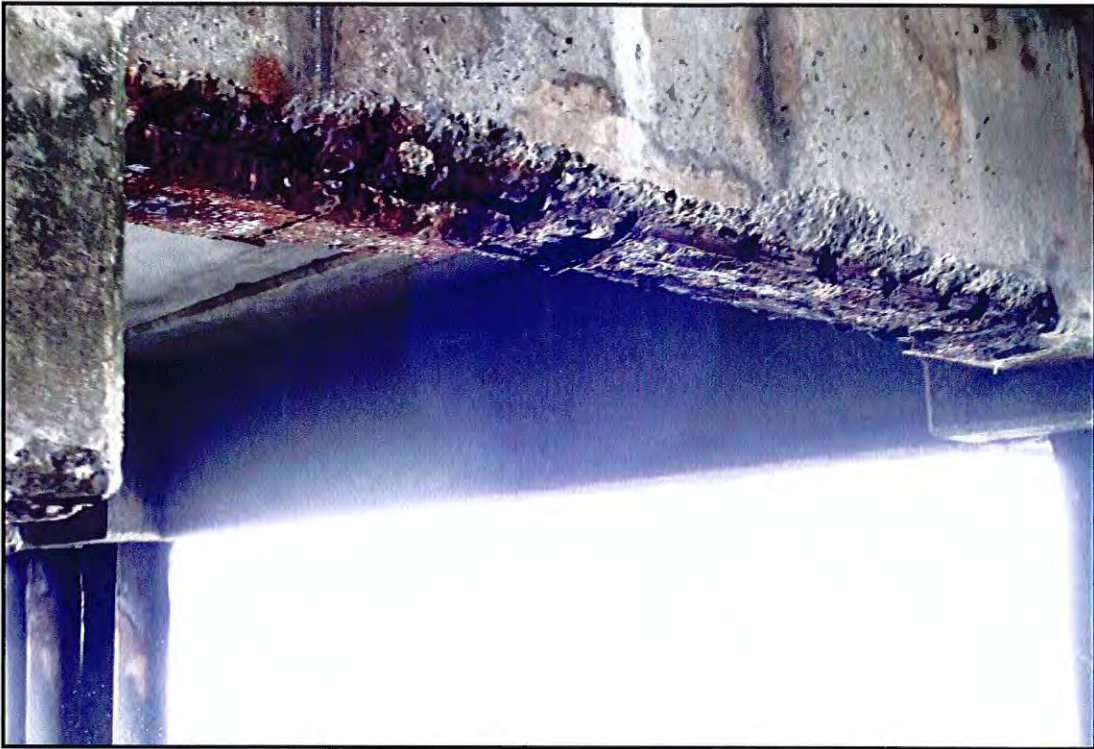
Photo B-27: Concrete beam in the Pier Shed with a full length spall and exposed reinforcement. View looking west at Bent T.5 and Pile Row 8-bar.
