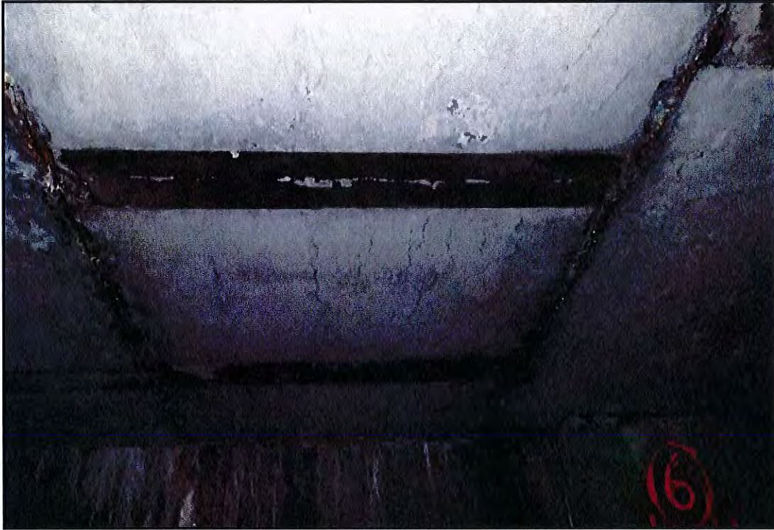
Photo B-33: Typical condition of Court Yard deck soffit with light shrinkage cracks. View looking west between Bent I and I-bar at Pile Row 9-bar.
