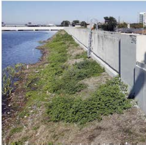
Floodwalls: Permanent or deployable walls used at the shoreline or upland to prevent flooding.
