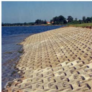
Revetments: Shoreline structures typically made of stone rubble or concrete blocks placed on a sloped surface to protect the underlying soil from erosion and reduce the force of wave action.
