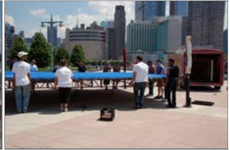
A glitch in the boxing ring assembly! The ring is six feet off the mark and must be moved.
